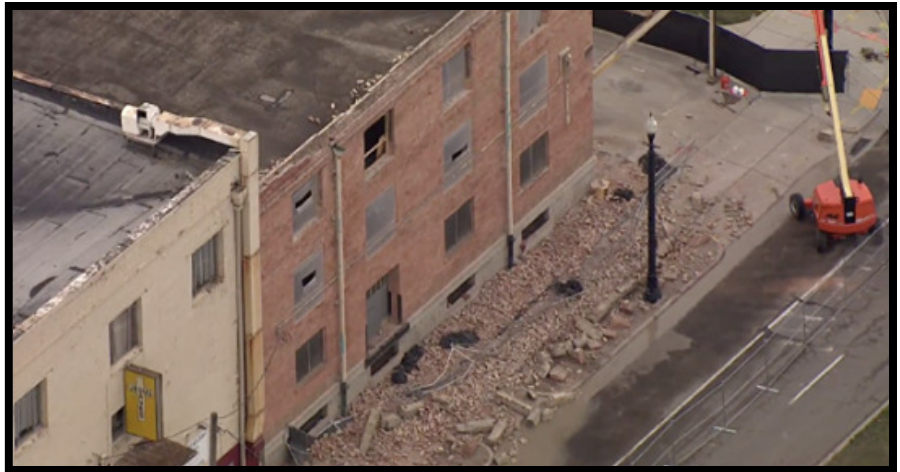
Earthquake damage in Magna
